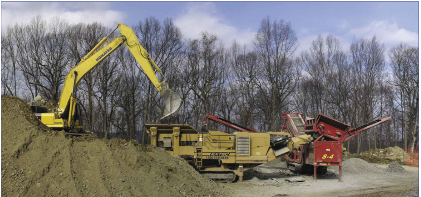
Construction of Peekskill's new state-of-the-art water treatment facility is already well underway. It will meet or exceed all federal standards and double the city's capacity, making it easier to accommodate future growth.
